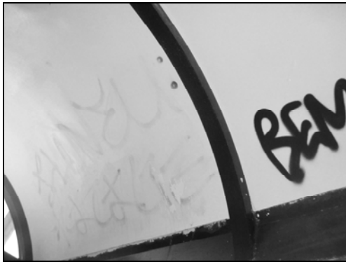
Graffiti on Interior Roof of Transit Shelter
