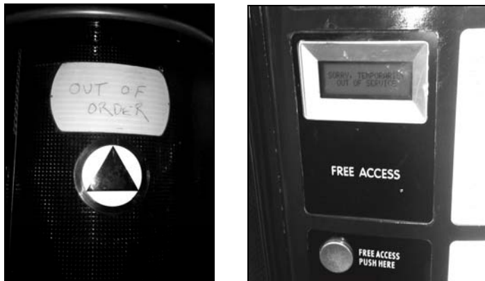
Figure 4.5 Photographs of Out of Service Public Toilets, Market Street
